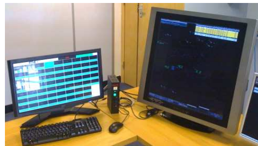
Warsaw ACC: Operational supervisors station.
