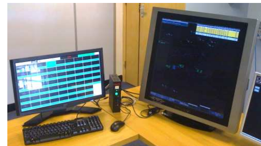
Warsaw ACC: Operational supervisors station.
