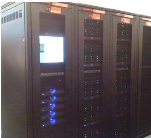
Sentinel video, audio and radar recording installation.
