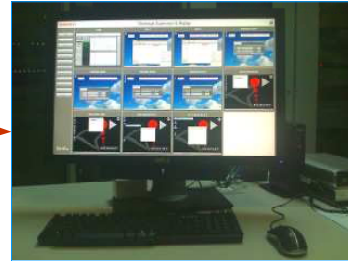
Technical Supervisor Real time remote control of Sentinel.
